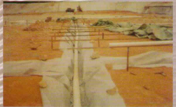
SUB-SOIL DRAINAGE PIPE
